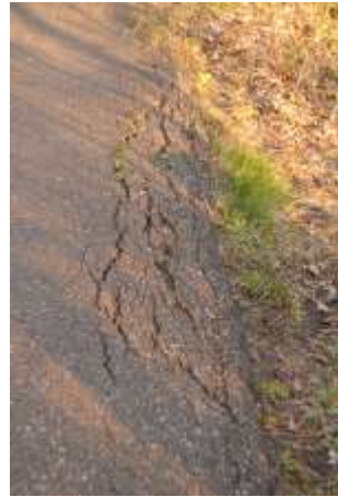
Water damage on trail over a natural drainage channel with no culvert
