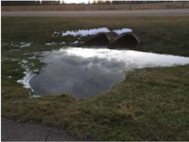
Trail is in between these road culverts and a wetland with no culvert under the trail
